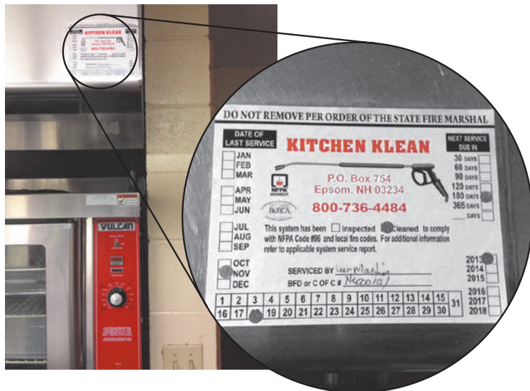
EXHIBIT 11.2 Certificate on the exterior of a hood.
