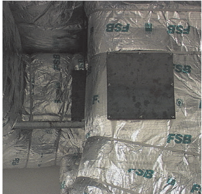
EXHIBIT 3.4 Example of a field-built grease duct enclosure. (Courtesy of Phillip Ackland Holdings Ltd.)
