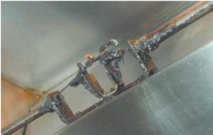
EXHIBIT 11.1 Fusible link requiring replacement.
