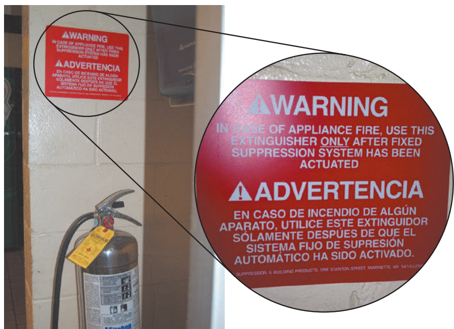
EXHIBIT 10.1 The placard required by 10.2.2 located directly above the fire extinguisher.
