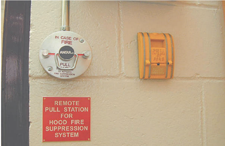
EXHIBIT 10.7 Example of a properly located manual pull station.
