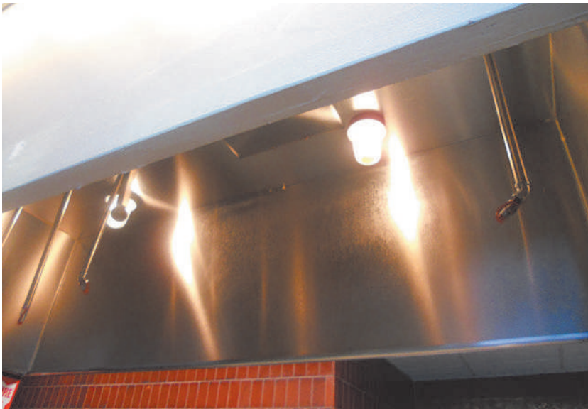
EXHIBIT 9.1 Lighting units in a hood.
