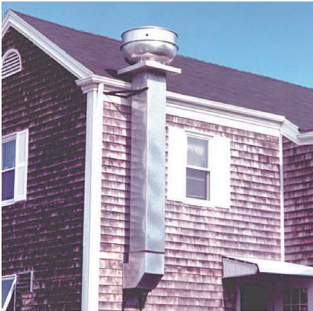
EXHIBIT 7.3 Exterior duct installation with questionable clearance.
