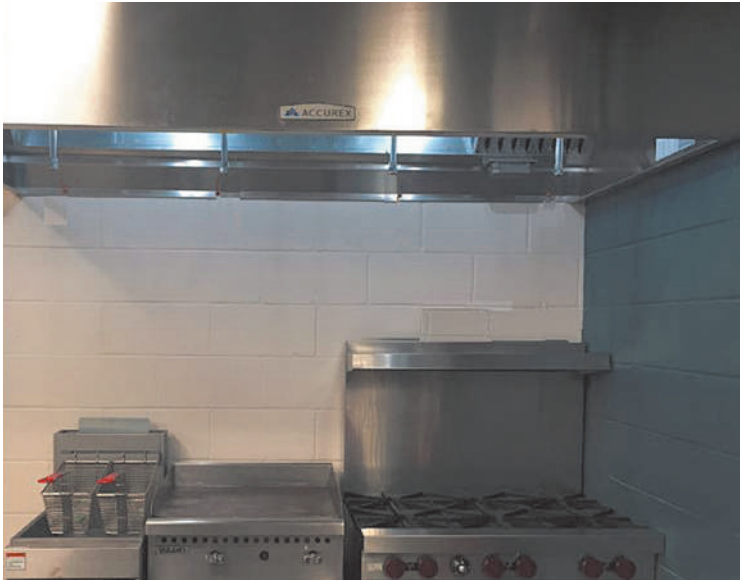
EXHIBIT 10.3 Hood suppression system. (Courtesy of Tyco Fire Protection Products)
