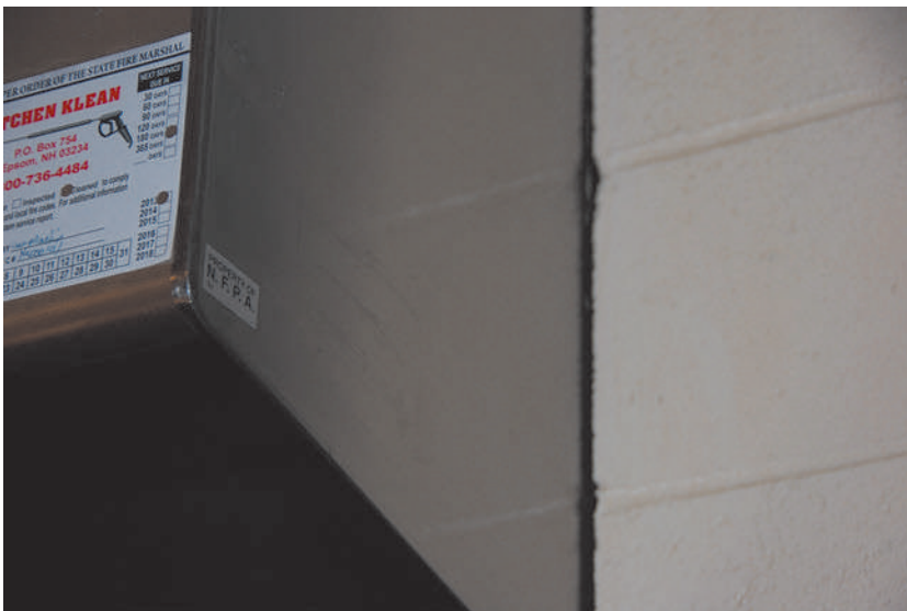
EXHIBIT 4.1 Example of near zero clearance to noncombustible construction.
