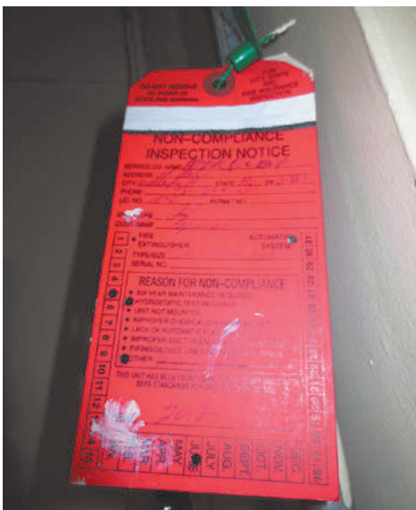
EXHIBIT 3.8 Example of a noncompliance tag.
