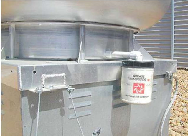
EXHIBIT 7.4 Grease collection container located near fan.
