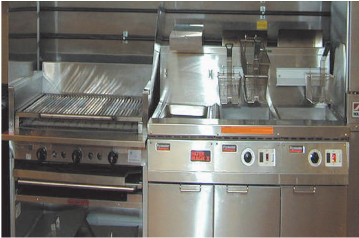
EXHIBIT 12.2 Example of separation between a fryer and surface flames provided by a baffle plate.
